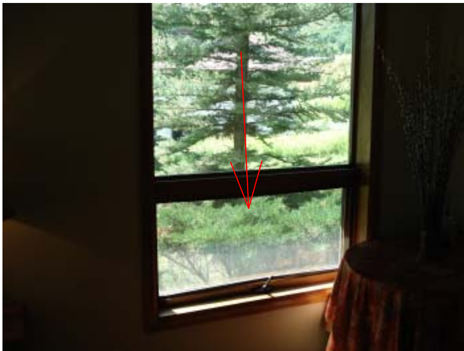
PIC 5: West facing awning window in the basement living room failed to open at the time of the inspection.
