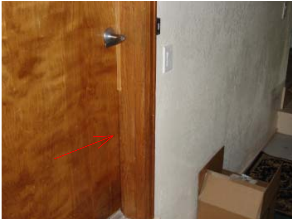
PIC 2: Door from garage to the interior has some damage to the door jam.
