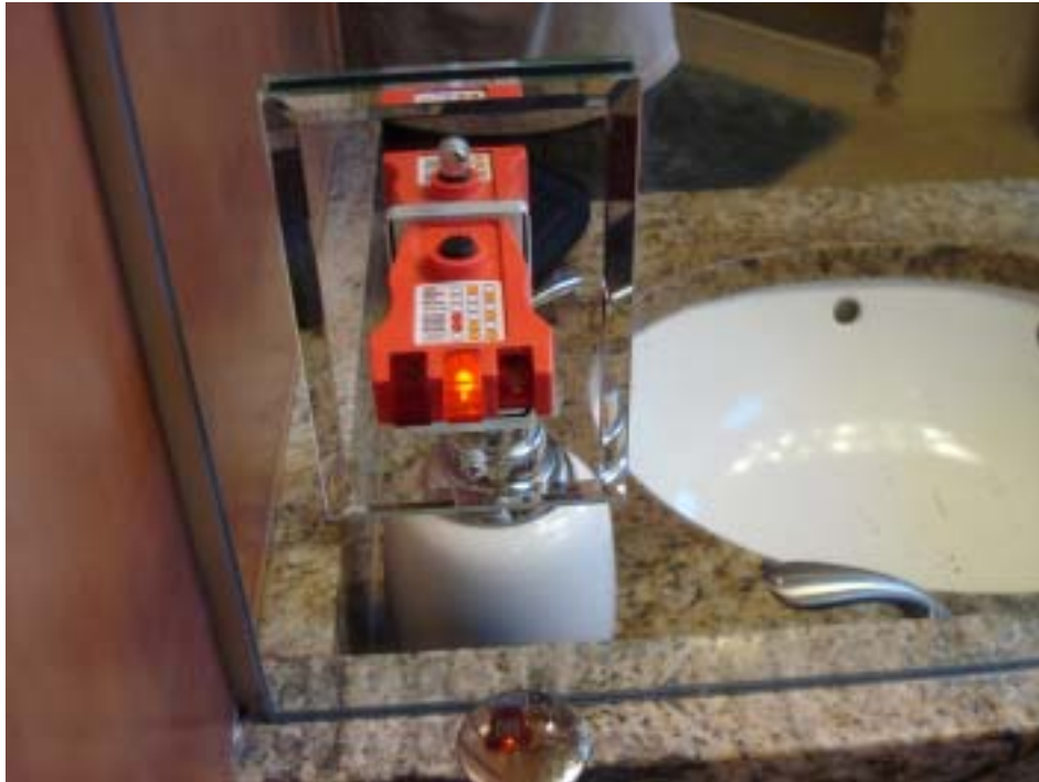
PIC 1: Open ground wire and defective GFI outlet in the master bathroom.
