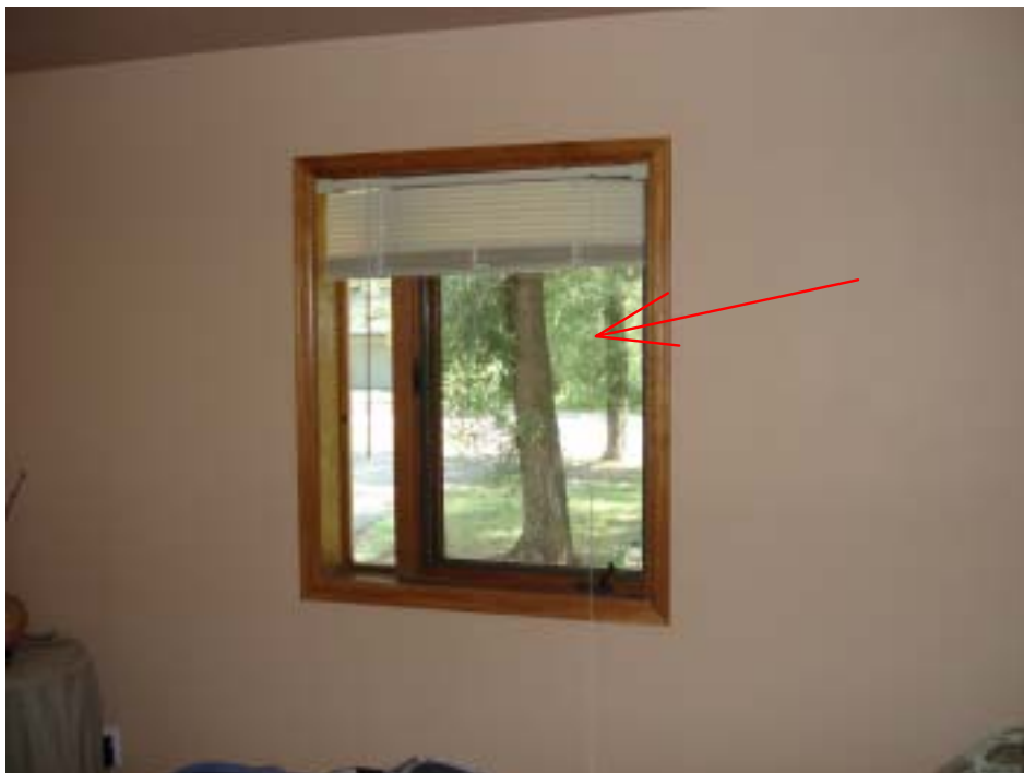
PIC 4: Casement window in the East basement level bedroom does not shut flush to the jam.
