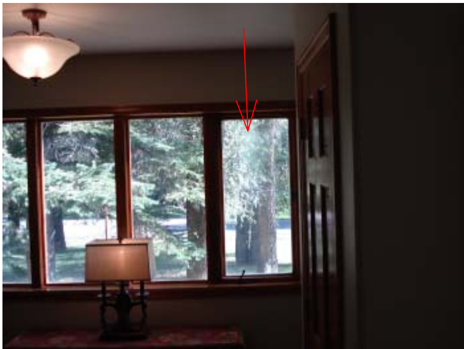
PIC 6: South facing basement casement window appears to have broken seals.
