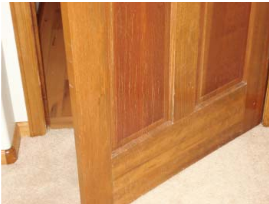
PIC 3: Surface damage to interior door (2nd level west bedroom).
