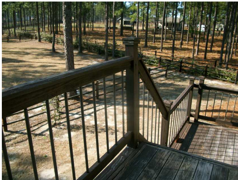
Loose handrails noted at the exterior stairs.
