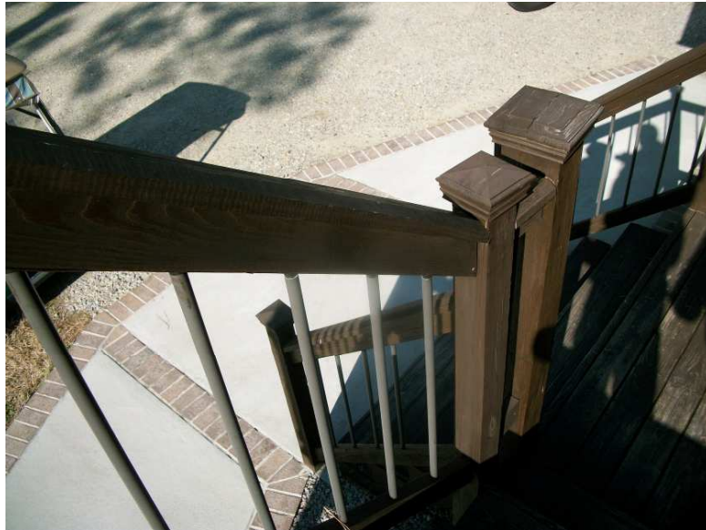
Damaged post caps noted at the exterior stairs.
